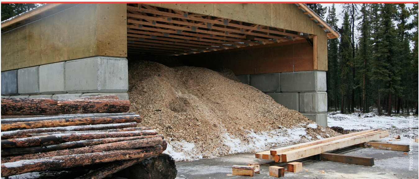
One-week supply of bulk wood chips for the biomass boilers at Teslin, Yukon
