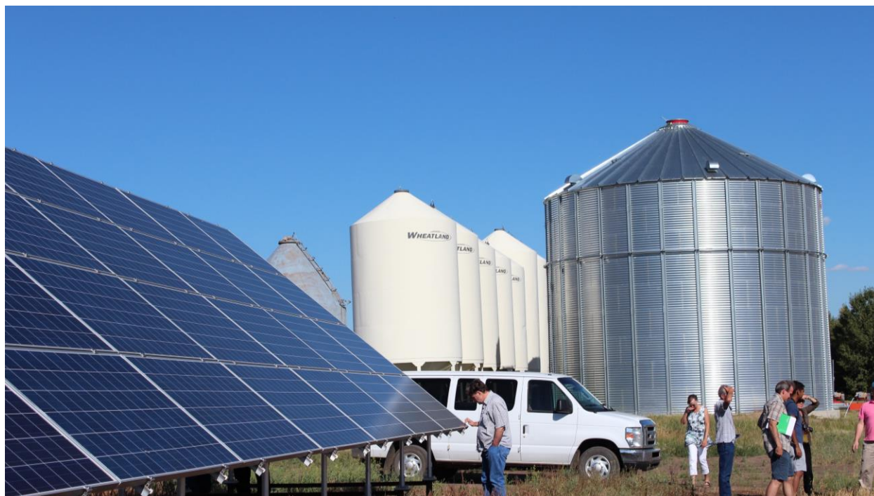
Solar installation on farm in Alberta
