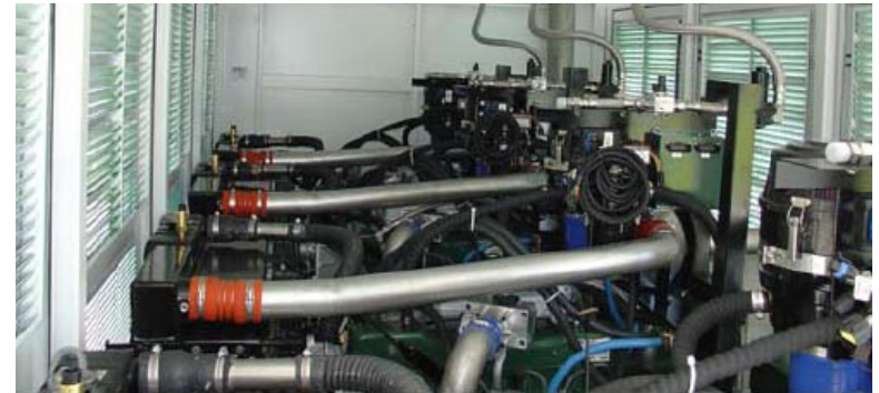
Interior View of HEC 250 kW H 2 Genset
