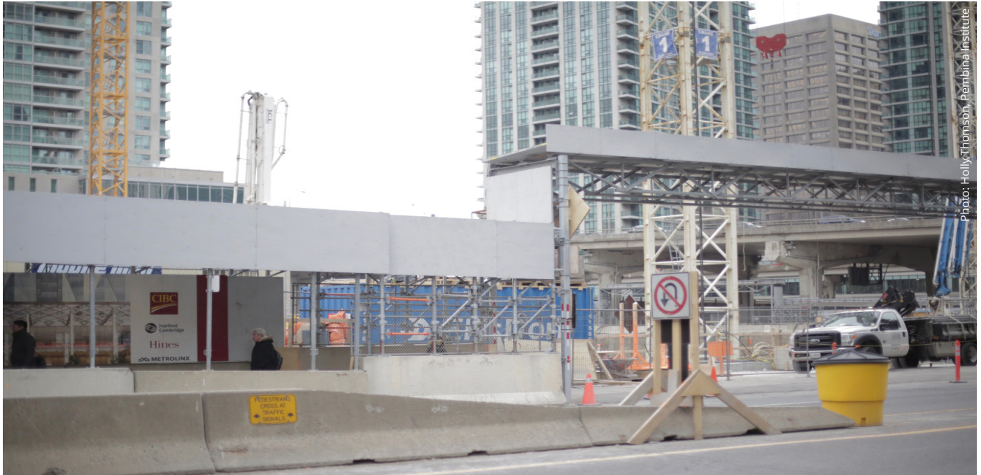
The future site of CIBC Square. Construction started in 2017 and is set to be completed by 2023.
