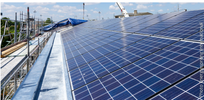
Solar PV can be installed as part of building retrofits.
