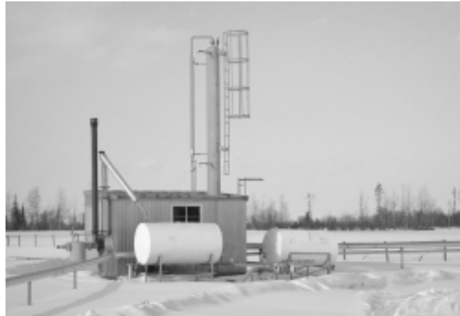
Dehydrator at well site
