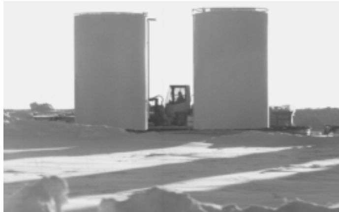
Tanks located within concrete dike.
