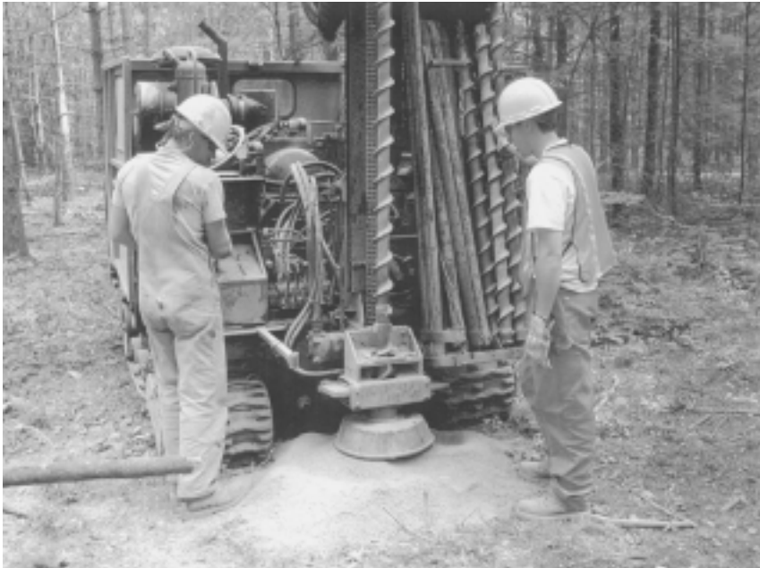
Workers use drills to create holes. They put explosives into the holes to make seismic waves.
