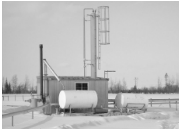
Dehydrator at well site
