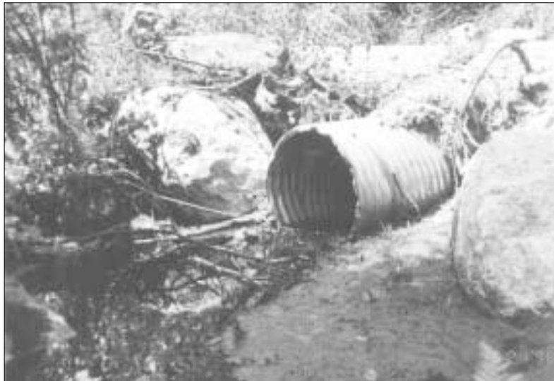
Licence holders have strong incentives to minimize the reported instances of non-compliance. The culvert above was not buried 10% in the streambed as required by the guidelines.
